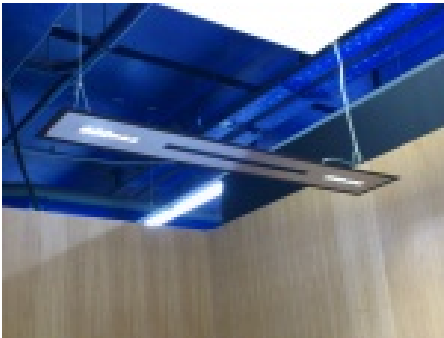
New lighting modules
